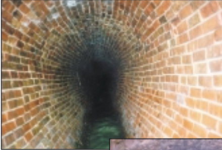
Deteriorated brick trunk sewer in Decatur, IL.
