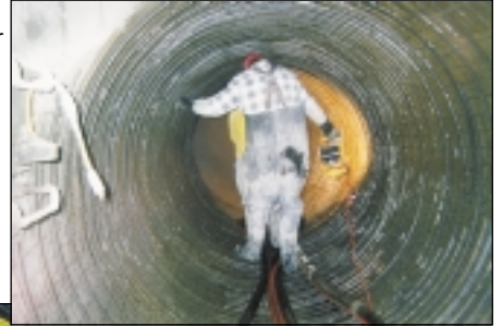
Welded wire mesh and rebar are placed in an extremely corroded trunk line.
