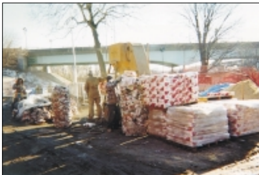
Batching of SewperCoat 2000HS for finish installation over the portland cement based underlayment.
