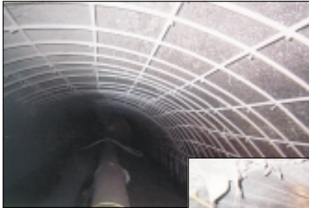
Deteriorated trunk line with reinforcing steel in place. Ready for the installation of the portland cement based underlayment.
