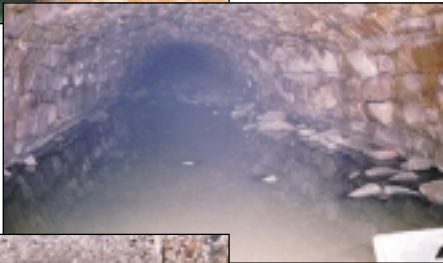
Corroded block trunk sewer in Pittsburgh, PA.
