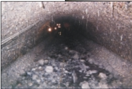
Failing concrete trunk sewer pipe in Philadelphia, PA.
