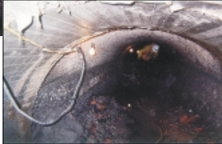
Deteriorated trunk line with the portland cement based underlayment installed.
